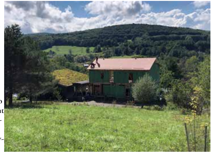
The Shelterbelt Barn rebuilt after a fire. Image provided by the author.
